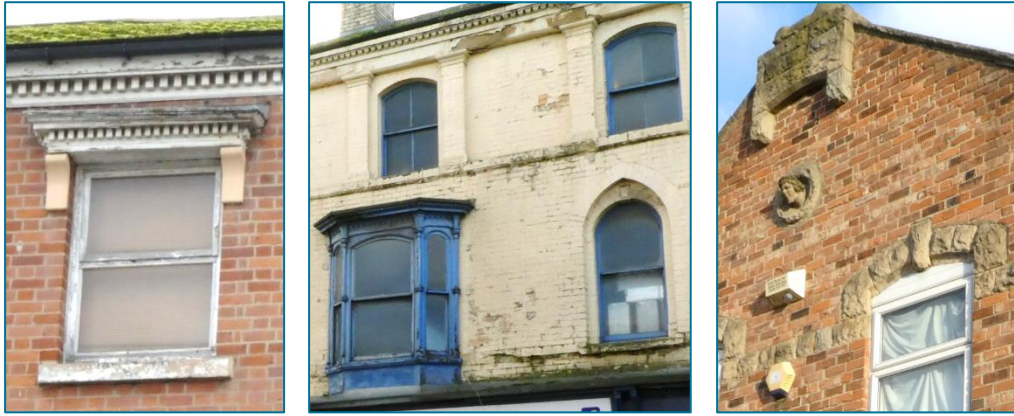
Left: Brick building with Italianate stone detailing to eaves and canopy above window. Centre: [E] Livingstone Building – All walling and detailing in brick, later painted; decorative bay window constructed in timber. Right: [F] 1 Leadenhall Street – Distinctive stone carvings by Robert Borrowdale (Photos © Gaby Rose, November 2023)
