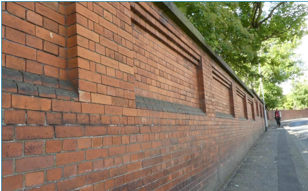
A5 – Top (Photo © Gaby Rose, February 2024): Hopetown underpass when approaching from Otley Terrace (west). The low walling to the left/west is also built in traditional brickwork with stone copings. Bottom (Photo © Gaby Rose, August 2023): Boundary walling along Whessoe Road with distinct recessed panels.
