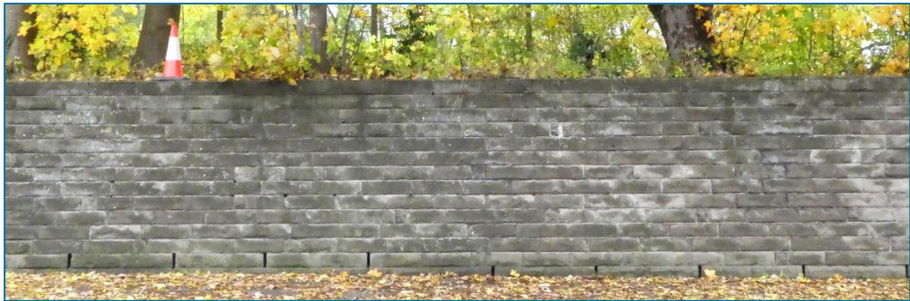
Coursed sandstone retaining wall along Hopetown Lane enclosing railway heritage site with mature vegetation behind. (Photo © Gaby Rose, November 2023)
